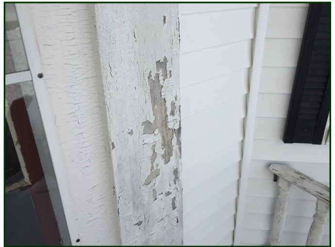
Photo #52: Photograph depicts general view of peeling/flaking paint on exterior trim
