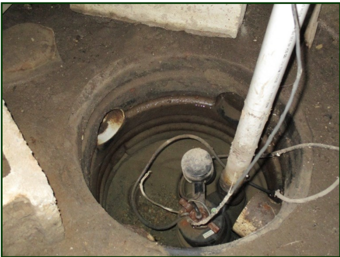
Photo #36: Sump pit with pump in southeast corner of basement
