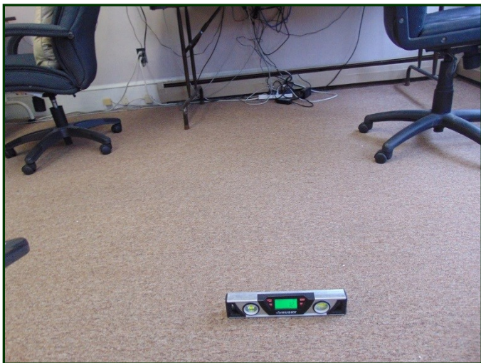
Photo #45: Measurement of sloped ground floor near northwest corner. The floor was sloped toward the west. Note digital level reads 1/2-inch per foot slope
