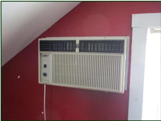
Photo #27: Through-wall air conditioning unit
