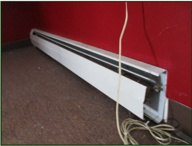
Photo #32: Fin tube baseboard radiator at attic level
