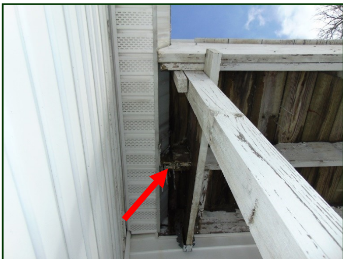
Photo #47: View of deteriorated fire escape framing on the west elevation.
