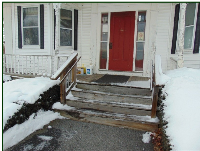
Photo #46: View of entrance steps on east elevation. Note porch is sloped away from the entrance.
