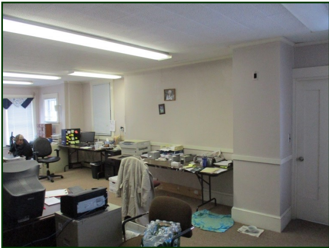
Photo #21: Office space with carpet flooring and surface-mounted fluorescent lighting fixtures
