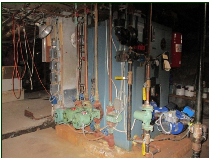
Photo #29: Gas-fired boiler in basement level
