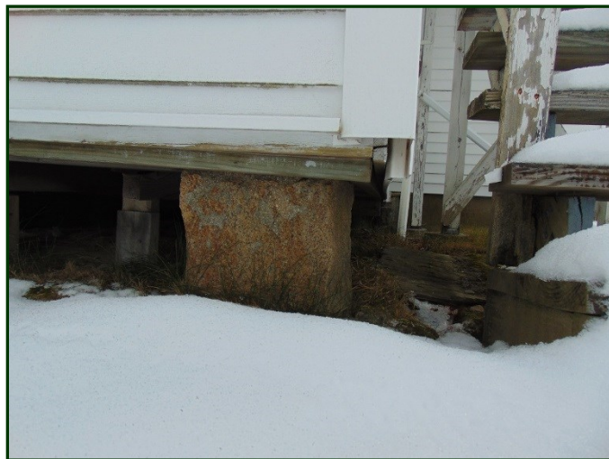
Photo #44: View of foundation block below northwest corner storage room. Floor in storage room was observed sloped toward west.
