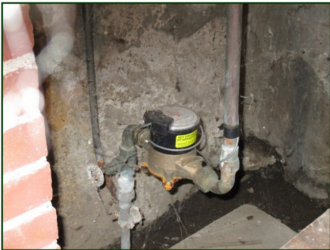
Photo #35: Domestic water service and meter in southwest corner of basement
