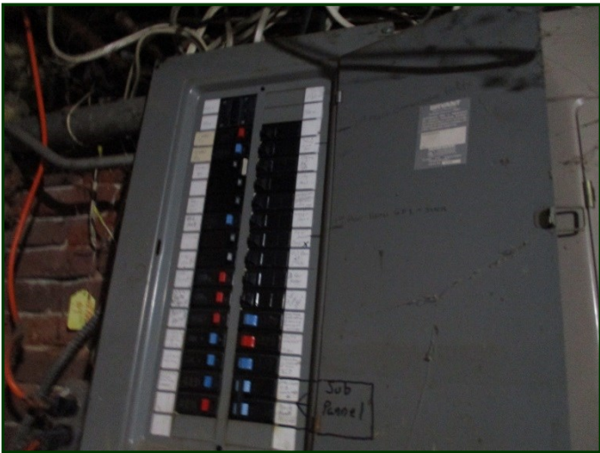
Photo #34: Main electrical service panel with circuit breakers in basement level
